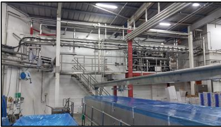
The compact HRS system sits on a platform above the curd production area
